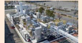
Hydrogen power generation facility (hydrogen CGS) constructed on Port Island in Kobe City
